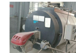
■ Air supply fan for boiler
